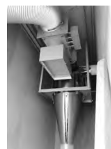
Fig. 2 A prototype silencer inside bran room
